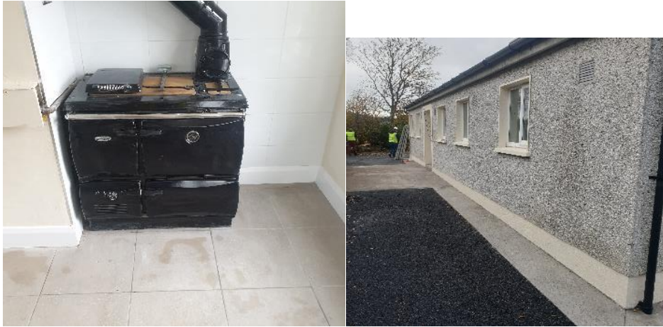
Major renovation works completed at traveller specific accommodation at Canal Drive, Ballinasloe
