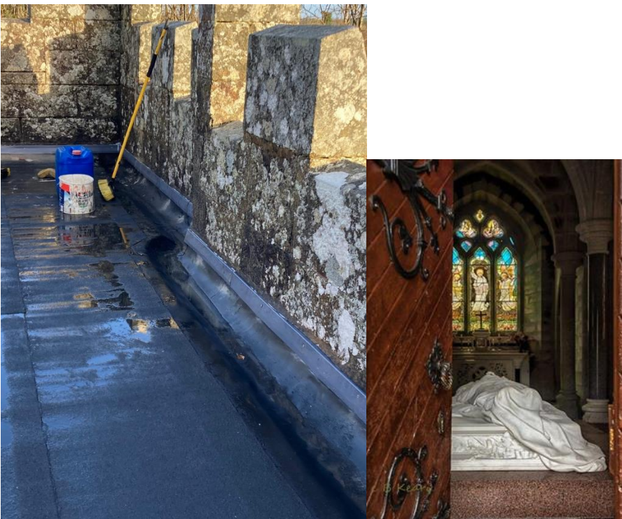
Repairs underway to roof of French Mausoleum, Monivea protecting the magnificent mausoleum and carved marble below
